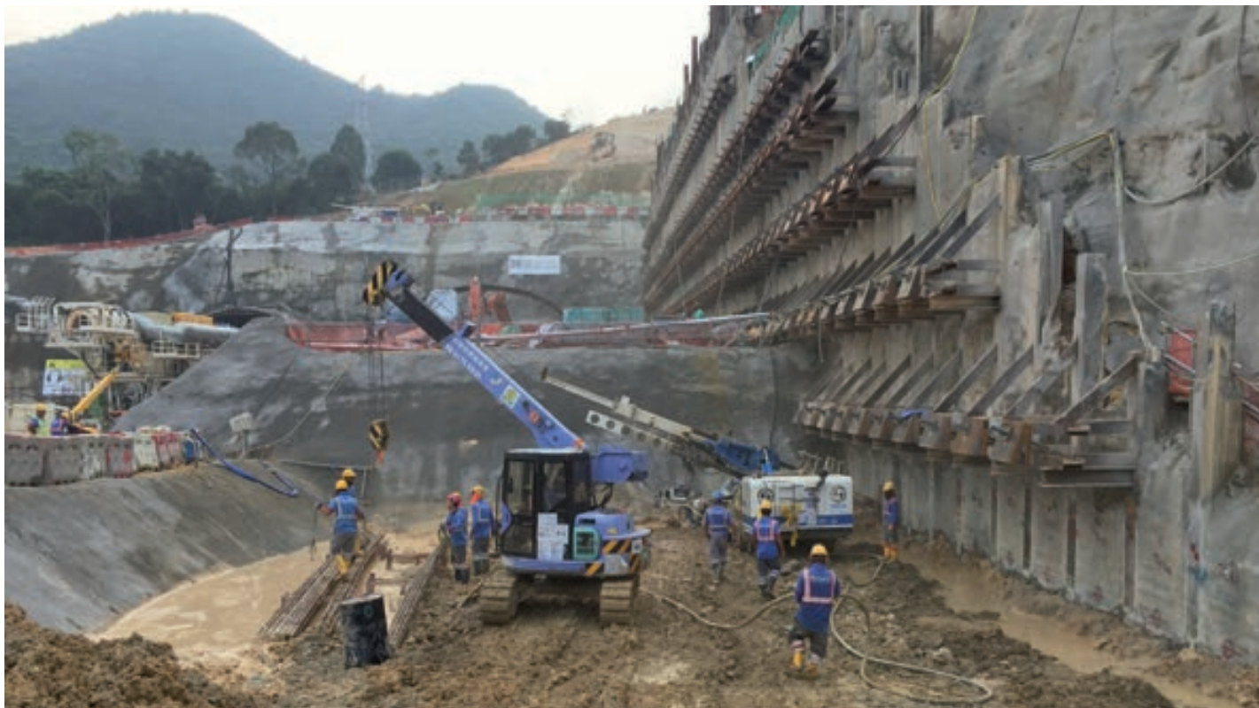
Lavori infrastrutturali per il nuovo "Liantang/Heung Yuen Wai Boundary Control Point". /Infrastructure works for the new "Liantang/Heung Yuen Wai Boundary Control Point".
