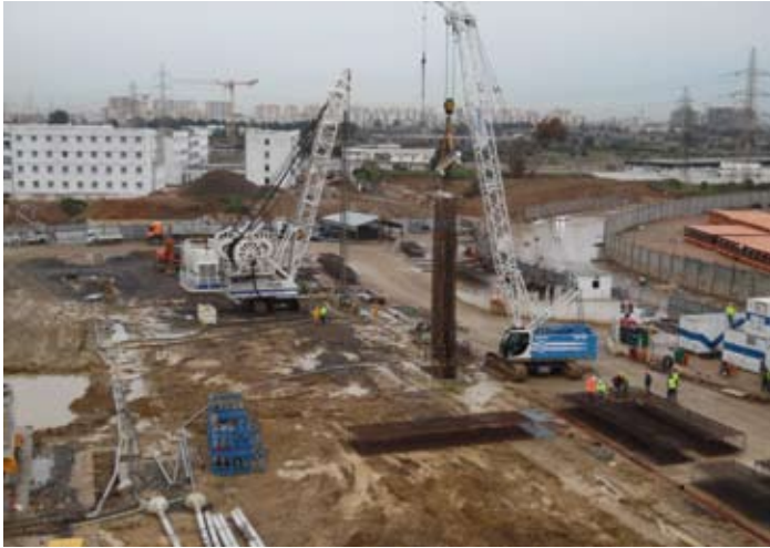
Metro Algeri - espansione El Harrach-Airport: Stazione Oued Smar Algiers Metro - El Harrach-Airport expansion: Oued Smar Station
