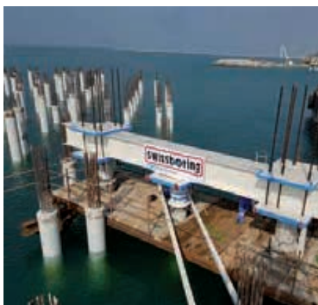
I pali in acqua realizzati da Swissboring. Piles in water made by Swissboring.
