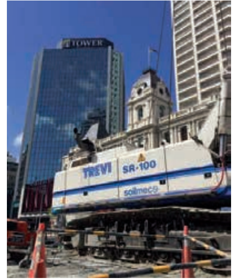
La SR-100 al lavoro ad Auckland. The SR-100 at work in Auckland.
